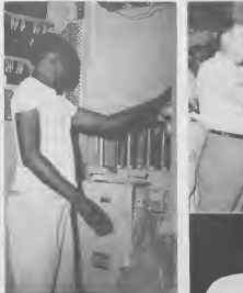
WHEN THE facilities of the substation had been checked out, the air circuit breaker on a Lago feeder was moved from its testing to operating position. OTRA CU e facilidadnan di e substation a worde checke, e interruptor di aire ariba un cable di Lago a worde movi for di su posicion di test pa posicion di operacion.
